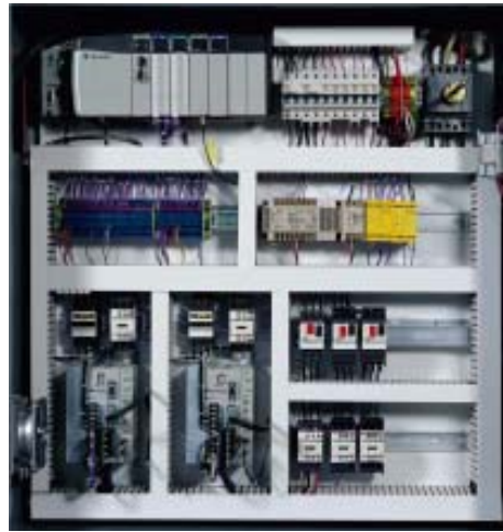
Allen Bradley PLC
